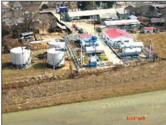
Moinesti Separation Installation
