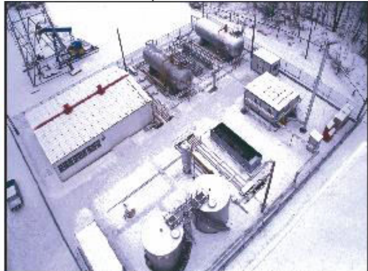
877 Mislea Separation Installation
