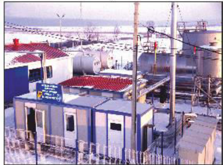
3 Dragomiresti Separation Installation
