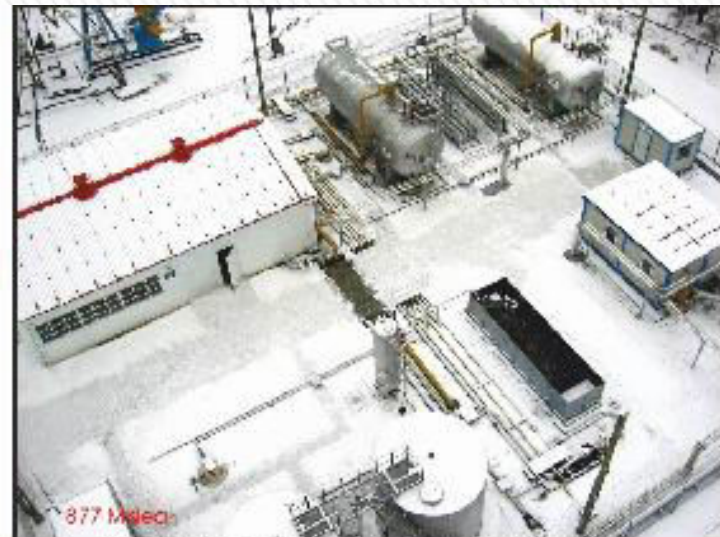
877 Mîlea Separation Installation
