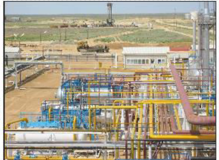
UKPG gas/condensate Separation Installation
