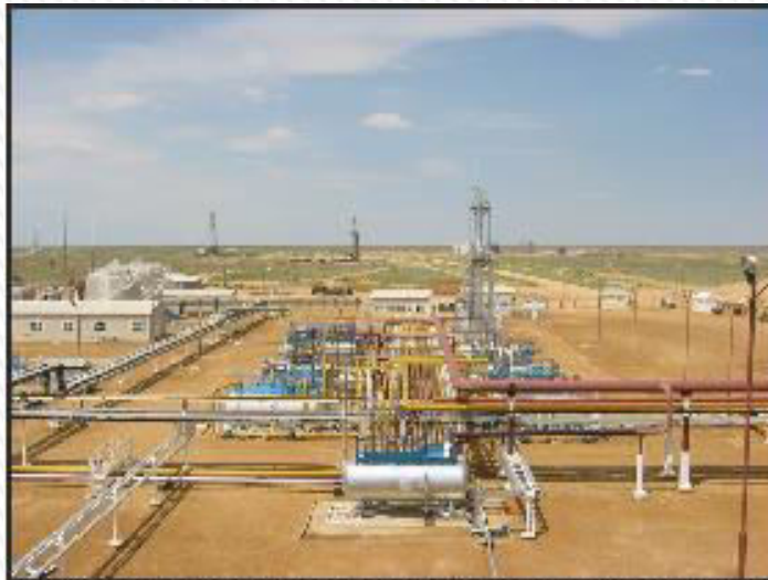
UKPG gas/condensate Separation Installation
