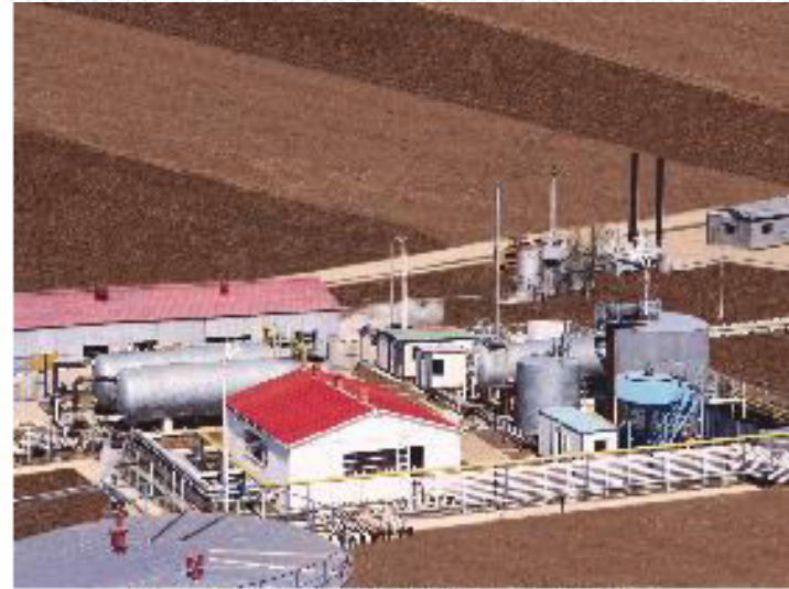
Craiova Separation Installation
