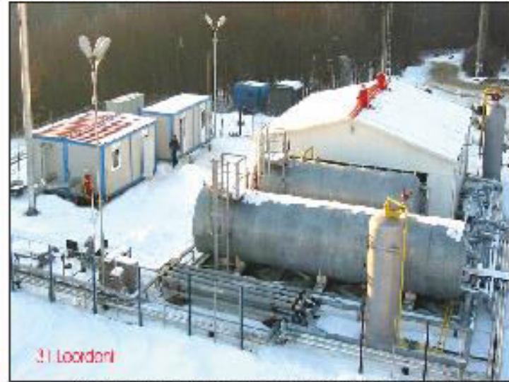
31 Leordeni Separation Installation
