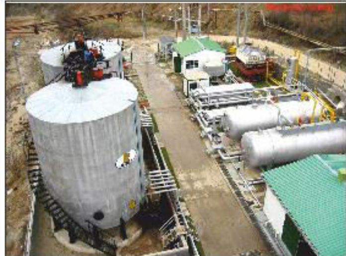
Predealu Sarari Separation Installation
