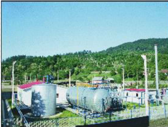
20 Tazlau Separation Installation
