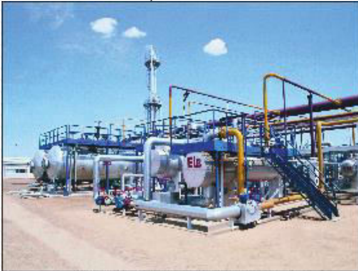
UKPG Separation Installation
