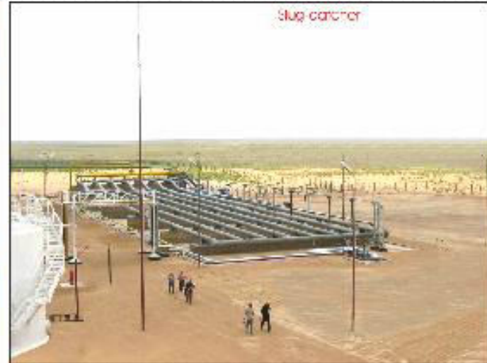
UKPG gas/condensate Separation Installation
