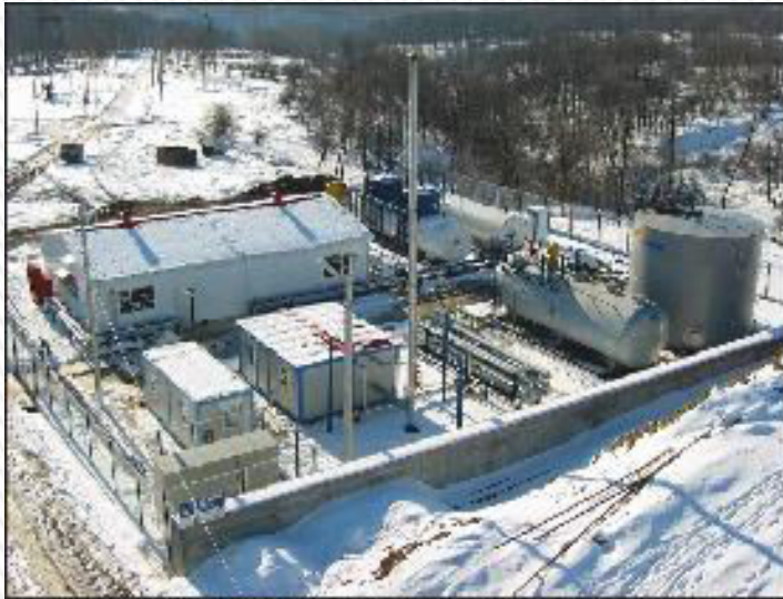
701 Gura Ocniței Separation Installation
