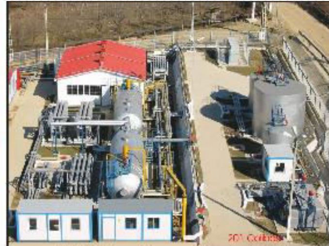
201 Colibasi Separation Installation
