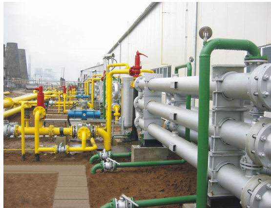
Ghercesti Electro-compressor Station-Heat exchangers
