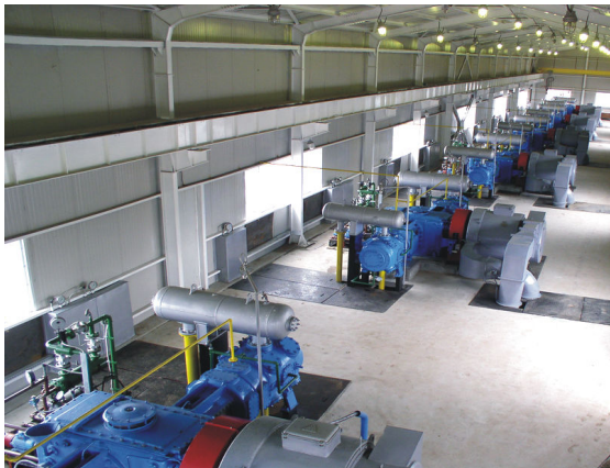
Ghercesti Electro-compressor Station(9 compressors)
