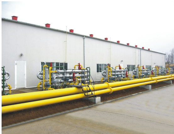
Ghercesti Electro-compressor Station-Heat exchangers
