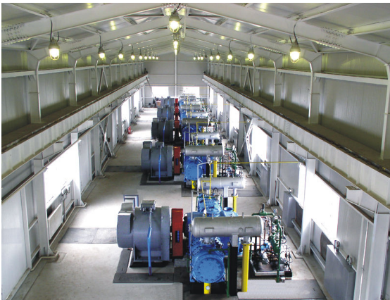
Ghercesti Electro-compressor Station(9 compressors)
